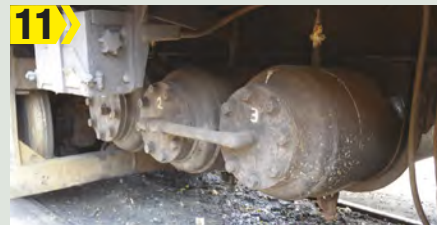
Fuel tanks and the battery box are tucked underneath the locomotive, but are very visible from the outside and so are worthwhile representing.
